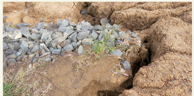
Image 1: Failure of a rock check dam in a sodic clay soil.
