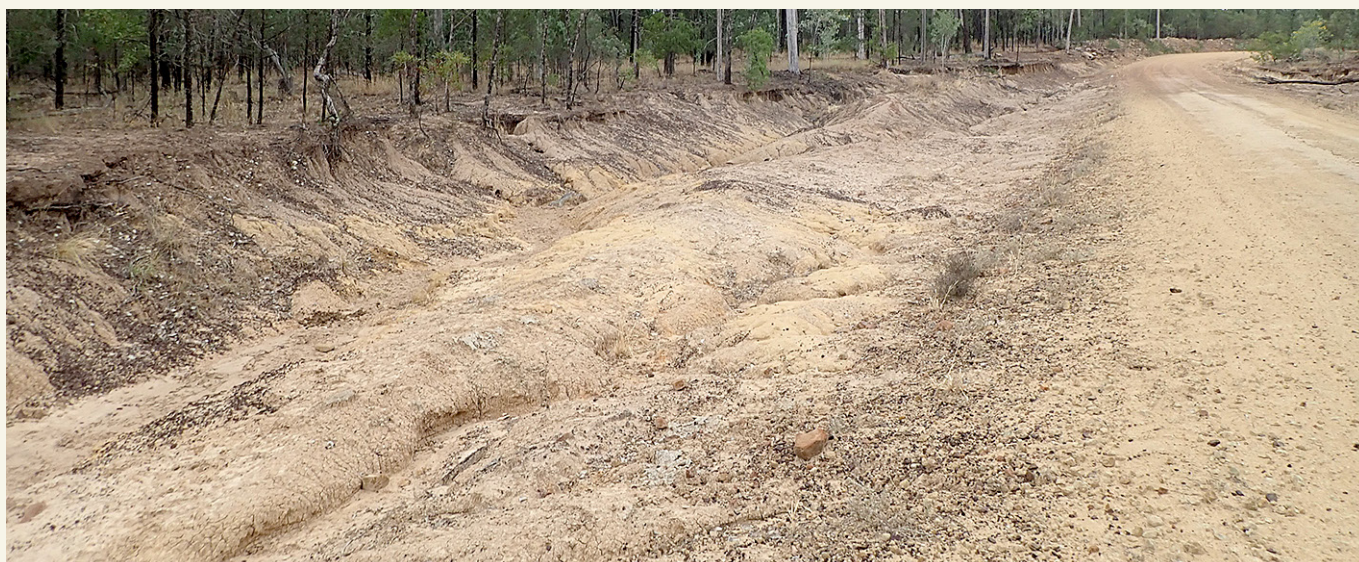
Image 2: Runoff from roads and tracks can lead to extensive erosion.
