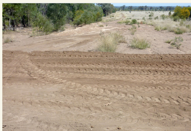
Image 1: Before and after whoa-boy construction. Note erosion to the left of the track in the before photo.
